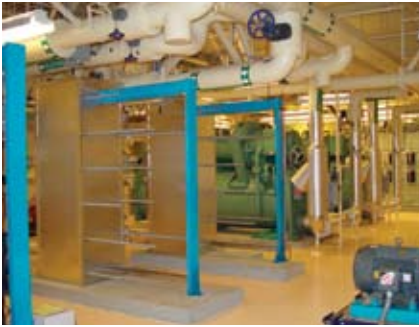
The FAA site in Anchorage now uses a groundwater cooling system that helps lower energy consumption as well as maintenance costs.
