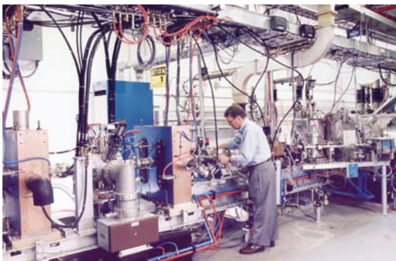
Continuous electron beam is injected into the accelerator tunnel
