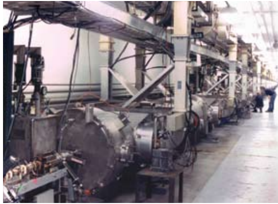
Cryomodules connected end-to-end around the accelerator tunnel
