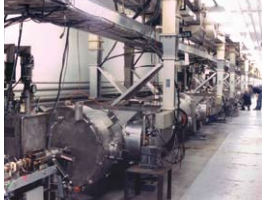
Cryomodules connected end-to-end around the accelerator tunnel
